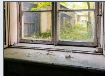
Window, Wall and Floor Damage
