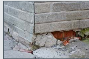
Foundation Damage & Basement Flooding
